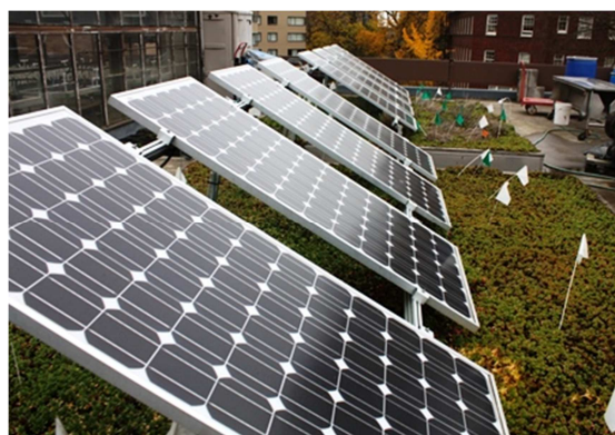
Figure 1. PSU Photovoltaic Test Facility
