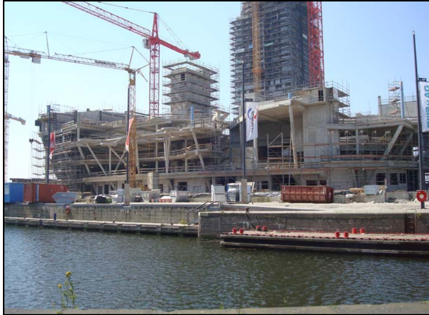
Figure 28: View of Klimahaus under construction in Bremerhaven (with high rise hotel in background).
