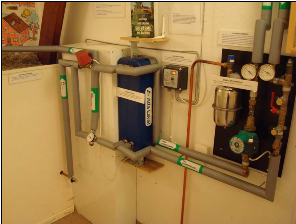
Figure 33: Solar hot water system at the Nacka Nature School, Stockholm.
